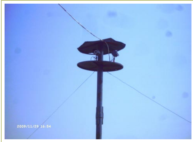
Figure 15: Short-range CCTV cameras installed by SSB to compensate for the shortage of men.
